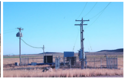
Transformers at Bowler Junction.
